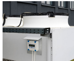
Heating/air conditioning/ventilation control
