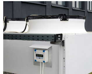
Heating/air conditioning/ventilation control
